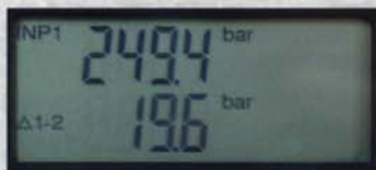
Pressure 1 Differential pressure
